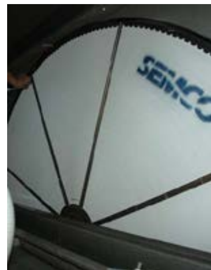
New 3 Angstrom Media Installed
