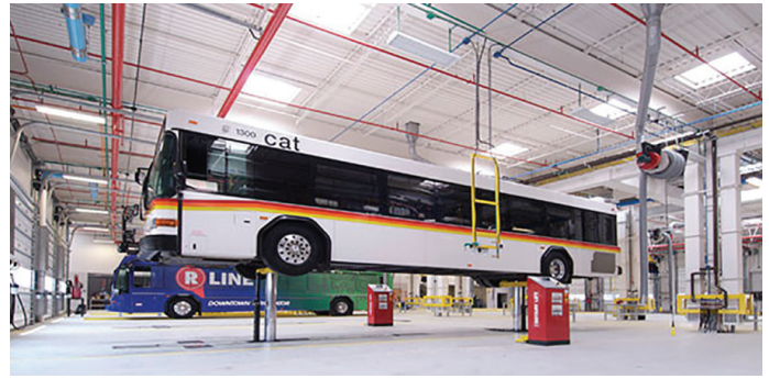
Mechanics in the maintenance facility enjoy year round comfort.
