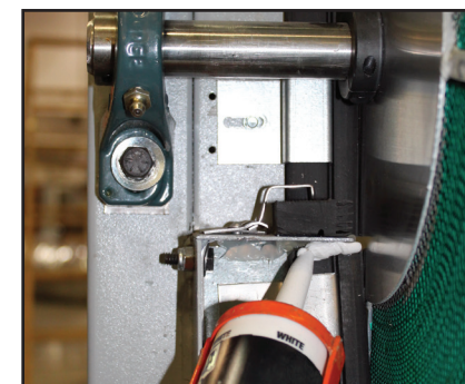
FIGURE 28. Caulk gap where purge seal abuts sheet metal end wall at the base of the purge.
