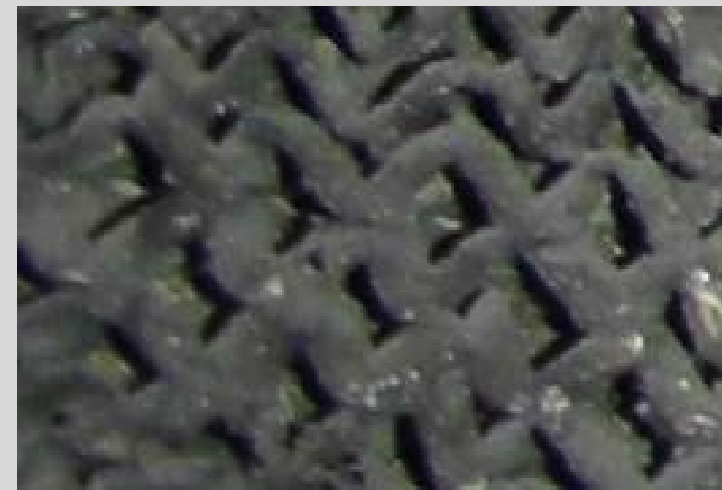
Corroded surface –no face coating
