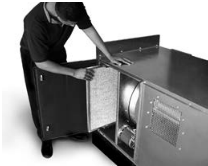
FIGURE 30. Replacing the return air filter.
